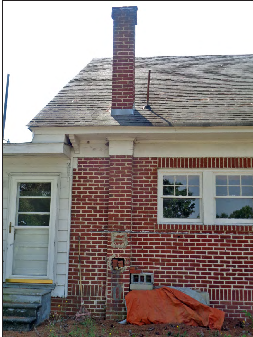
PLATE 9: 655 Longbranch Road Dwelling Damaged Rear Chimney and Addition Door, Looking Southeast
